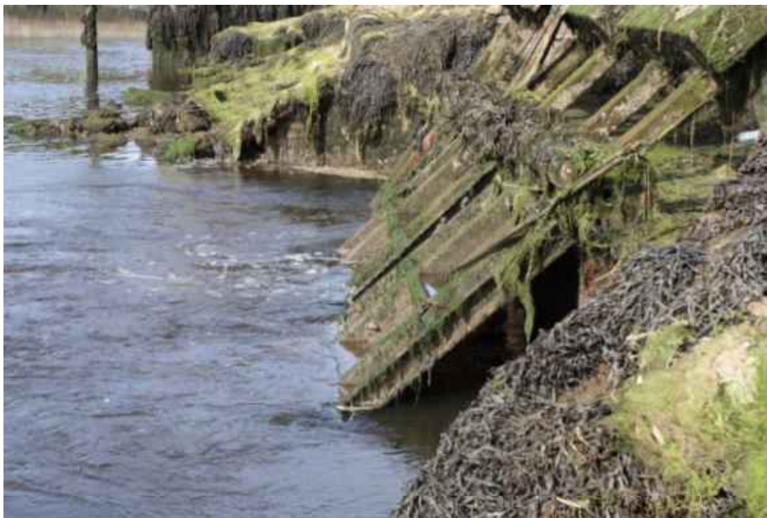
Figure 3.12. Counter-weighted tidal flaps on the Lyminster River, Hampshire. These tend to open further and remain open longer than conventional flaps of similar weight.
