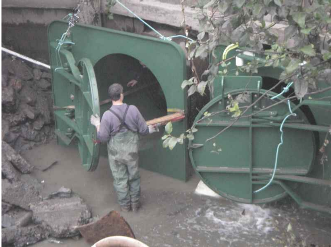
Figure 3.9. Side hinged gates being fitted to replace top-hung flaps at Schneider Creek, Washington State, USA. The issue here was passage of coho salmon. The right-hand gate is fitted with a Muted Tidal Regulator (see Section 4.4). Photograph courtesy of Tom Slocum, Washington Conservation Districts NW Region Engineering Program.
