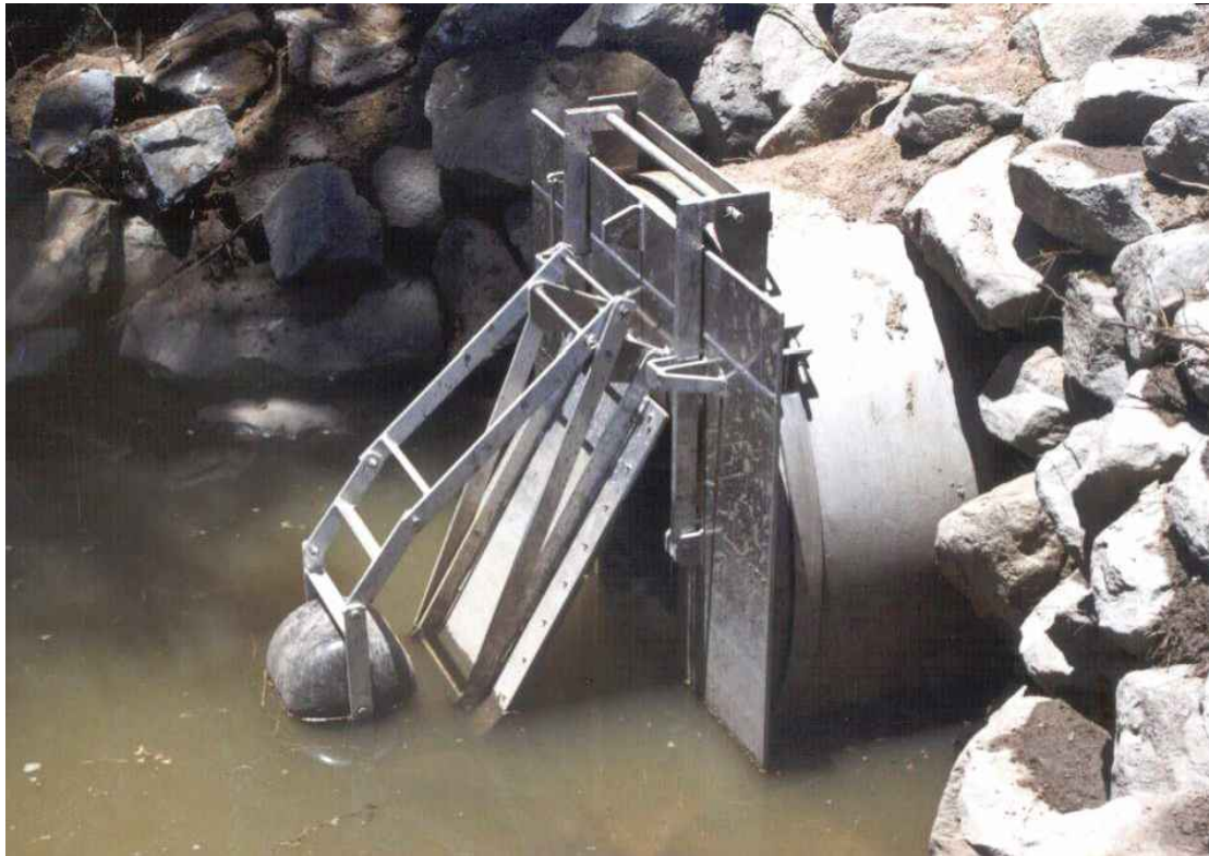
Figure 4.2. Automatic tidal flap in New South Wales, Australia. From Green and Pease (2007).
