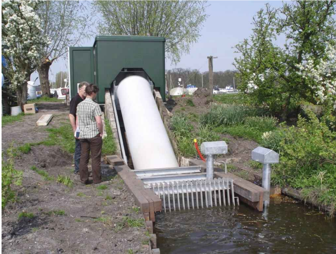
Figure 5.10. Fish Flow Innovations Archimedes screw pump at a pumping station at Zwanburgerpolder, Netherlands. Photograph courtesy of Fish Flow Innovations.
