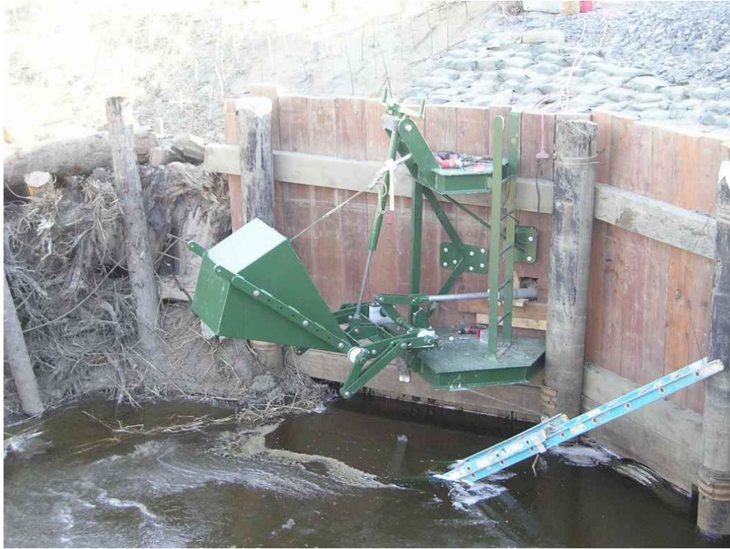
Figure 4.6. Float mechanism for an MTR gate at Schneider Creek, Washington State, USA. Photograph courtesy of Tom Slocum, Washington Conservation Districts NW Region Engineering Program.
