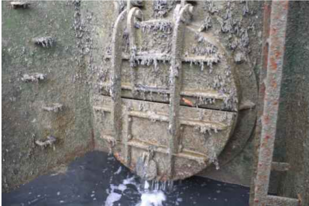
Figure 3.15. Tidal flap at Maydays Farm, Essex. This is an interesting installation as the flap is separately hinged in two halves, and the lower half is fitted with a small “cat-flap”, presumably designed to operate at very low flows. However, in this case the construction of the cat flap is too heavy (cast iron) to really be a useful contribution to elver passage.
