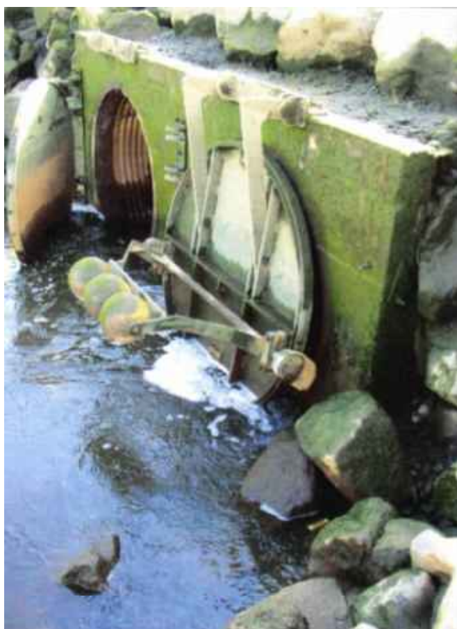
Figure 3.24. The nearer flap is fitted with a Mitigator Fish Passage device, which holds the door ajar until the rising tide lifts the floats. The further culvert has a side-hinged gate, converted from a top-hinged flap – the remains of the flap hinges can be seen on top of the concrete bulkhead. Photograph courtesy of Guillermo Giannico, Oregon State University.
