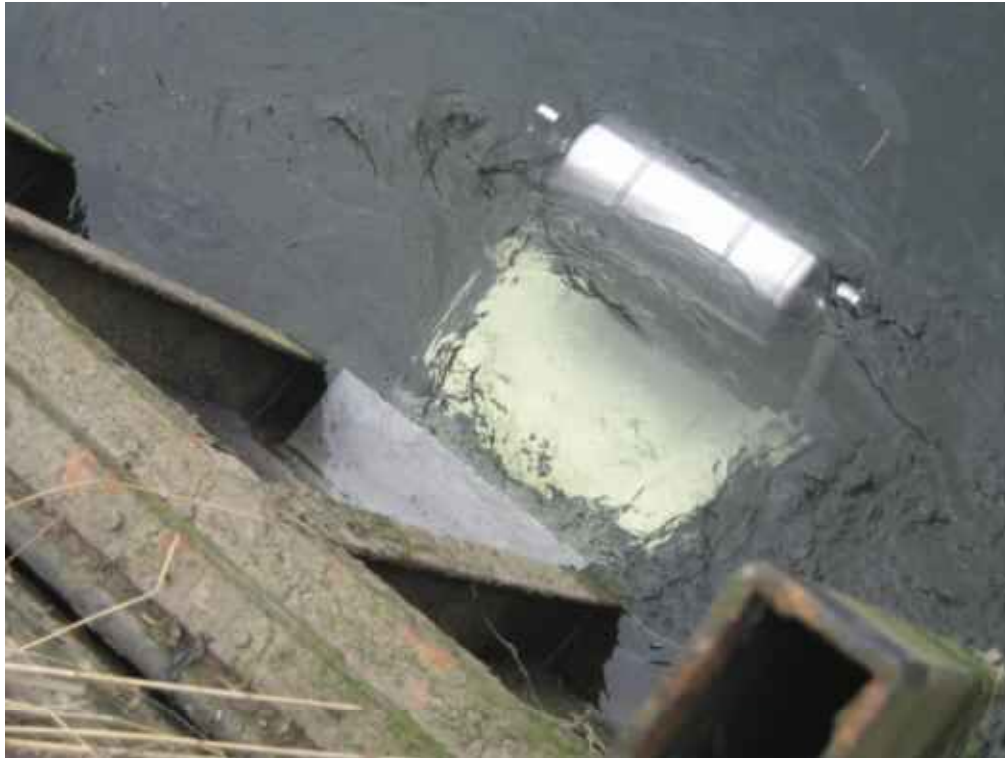
Fig 3.18. Bottom-hinged cat flap in tidal flap on the River Stiffkey in an open position, with the float being lifted by the tide. As the tide rises further, the flap will close. The dimensions of the opening are 600 x 300 mm. Photograph with permission of Ros Wright, Environment Agency.
