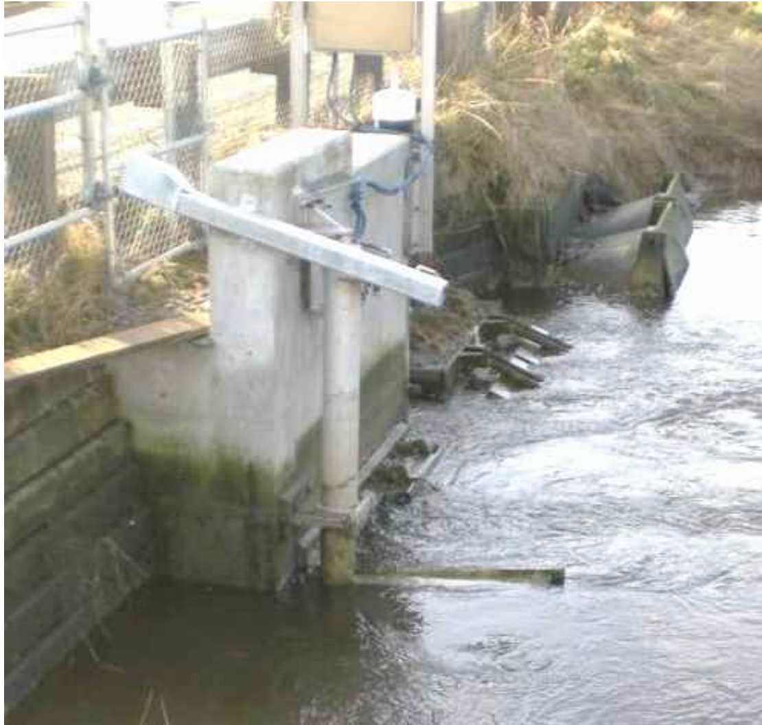
Figure 4.8. Juel Variable Backflow Flap Gate (VBFG™). The gate is fully open, on the ebb tide. Photos reproduced with permission from Juel Tide Gates of Seattle, Washington, USA ( www.jueltide.com ).
