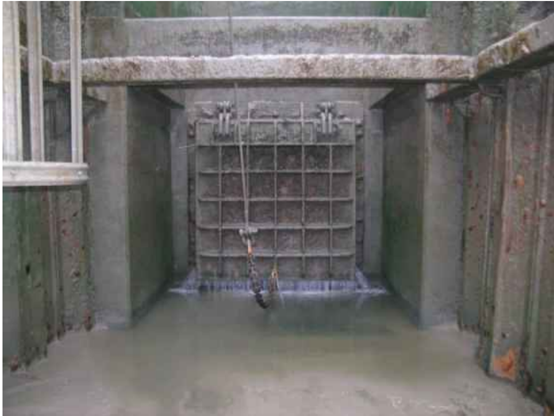
Figure 3.14. Two metre square section tidal flap at Havering, Essex, draining an area of Havering Marshes to the Thames Estuary. Although this was not the intention, the weight of the chain and cable effectively reduces the closing weight of the door, delaying closure. Additional weight would hold the flap open beyond level equalisation on the rising tide.
