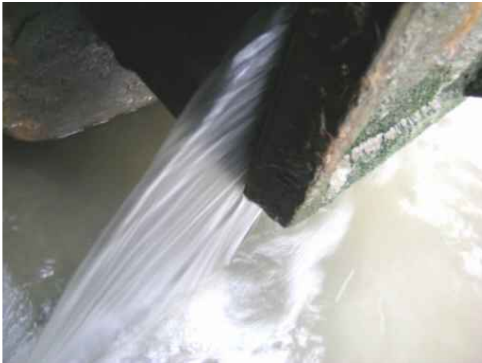
Figure 3.6. Water squirting through the gap of an almost-closed rectangular tidal flap at the mouth of a marsh drainage channel on the Thames Estuary. Even when the tide rises to the bottom of the door, this flow is too fast for eelers to overcome. As the tide rises past the bottom of the door and the velocity starts to fall, the gate shuts.
