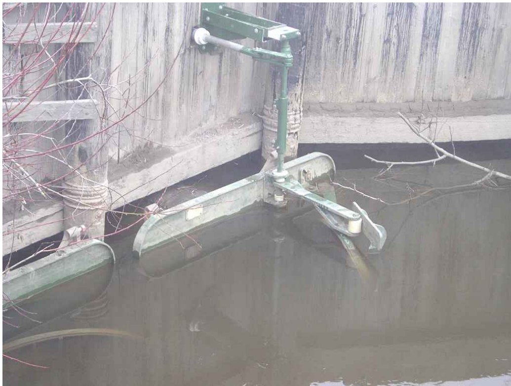
Figure 4.7. Gate actuating mechanism for an MTR gate at Schneider Creek, Washington State, USA. The door is being held open. This is the right-hand door in Figure 3.9. Photograph courtesy of Tom Slocum, Washington Conservation Districts NW Region Engineering Program.
