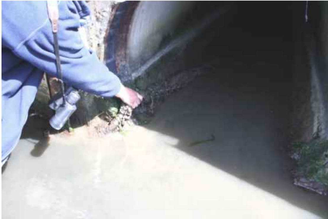
Figure 3.23. Chain wrapped in garden mesh laid through a culvert at Lodmoor. The chain extends through the tidal flap at the seaward end of the culvert (Figure 3.21), and is anchored to a stake in the stream bed.
